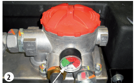
Clogging indicator on the hydraulic oil filter
