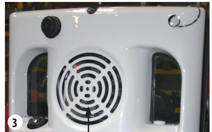
Air conditioning condenser
